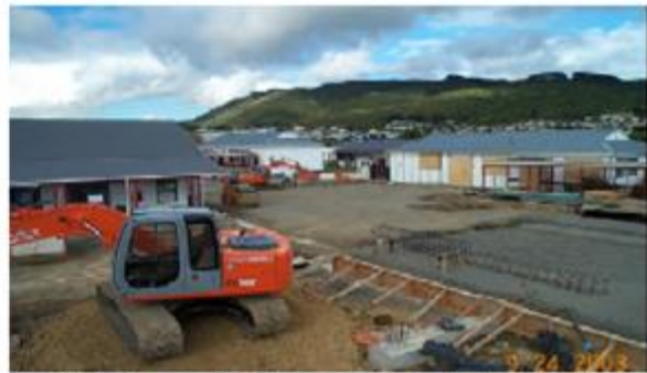
4. With formwork and reinforcing steel put in place the building floor is ready for concreting.
