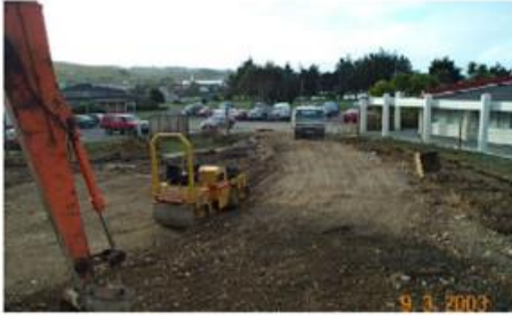
1. A temporary road is created to allow access onto the construction site.
