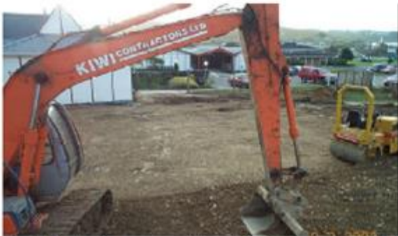
3. With drainage complete, shingle back-fill is laid to create a platform for the new building.
