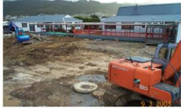
2. Essential drainage works in the foundations of the new building gets underway.
